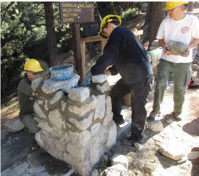
Alex Mills had a crew at Red Box to work on the stone pilasters, and they successfully completed the reconstruction of the pilasters for the trailhead into West Fork Canyon
