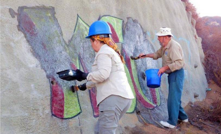
Peter and Lauren covering up graffiti on Mt. Lowe Road. Photo by Brenda Beck
