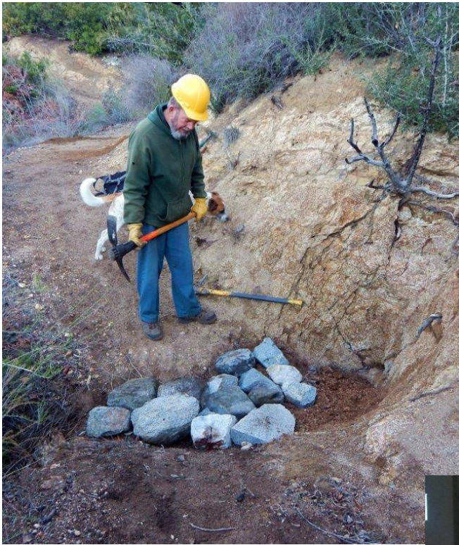
Peter installing a French on the Trail Canyon Road by Brenda Beck
