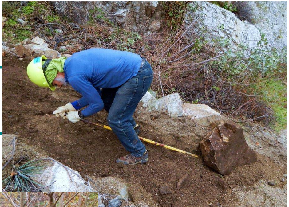
Dave Baumgartner moving a rock off the Trail Canyon Road by Brenda Beck
