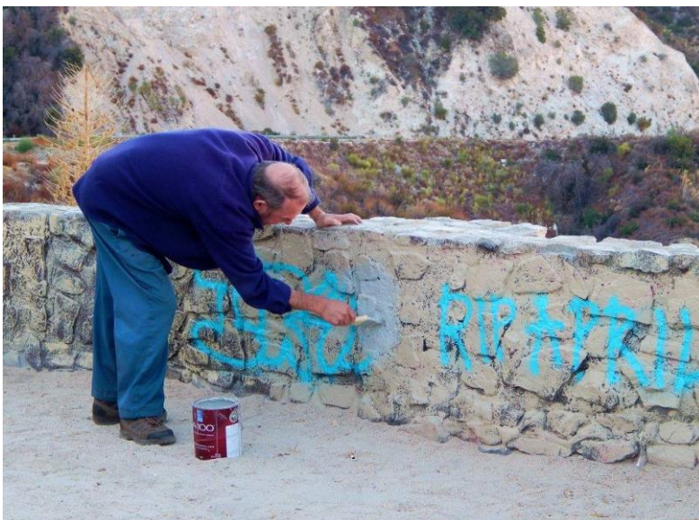
Volunteer Peter Harrison painting over graffiti at the Big T Reservoir Lookout by Brenda Beck
