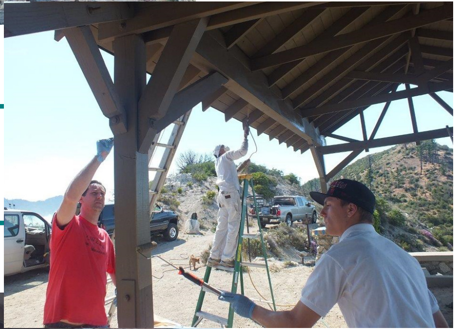
INSPIRATION POINT repairs by SCENIC MT. LOWE RAILWAY crew By Brian Marcroft
