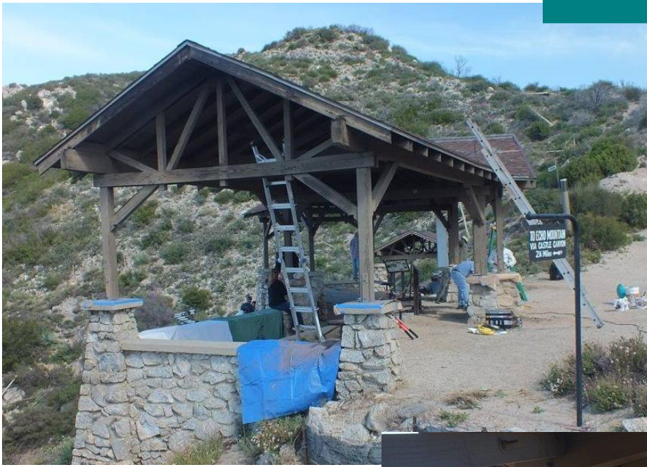
INSPIRATION POINT repairs by SCENIC MT. LOWE RAILWAY crew By Brian Marcroft
